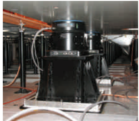
STACIS® 2100 on a "riser" installed under a TMC platform in a 36" tall raised floor
